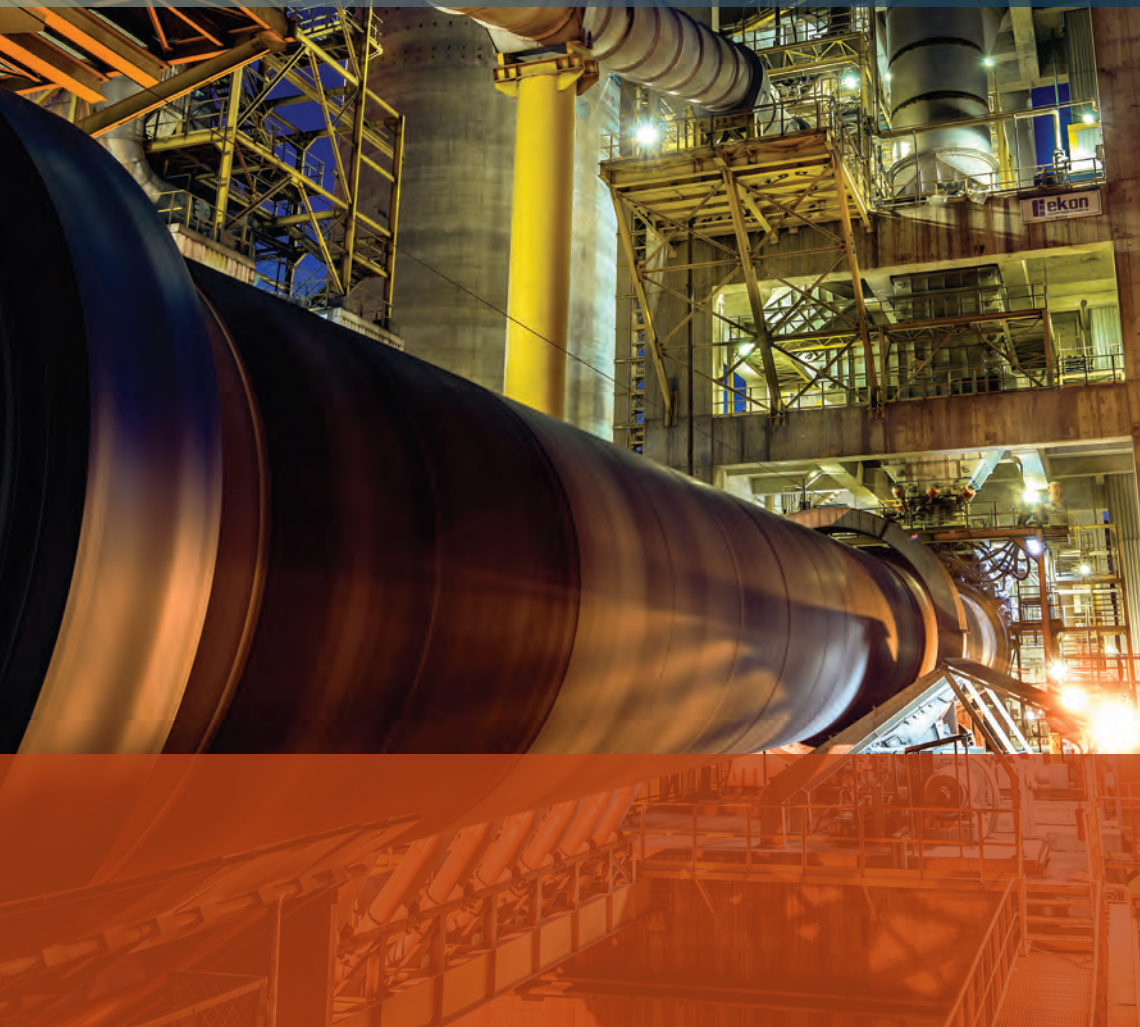
Overview of clinker rotary kiln with preheater tower at the back
